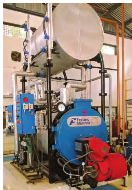
Forbes Marshall Energy Efficient Lab
